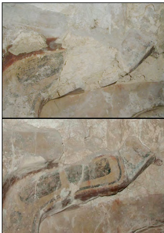
Re-adhesion of polychrome-modeled stucco fragments by using autogeneously air-setting mortar. Calakmul - Mexico.
